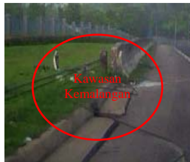
Photo 3: The rigid steel post beside the concrete barrier at MRR2 near Kepong Metropolitan Park.
