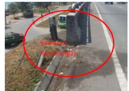
Photo 4: The rigid steel post beside the bridge parapet concrete barrier at Lebuhraya Jelutong.
